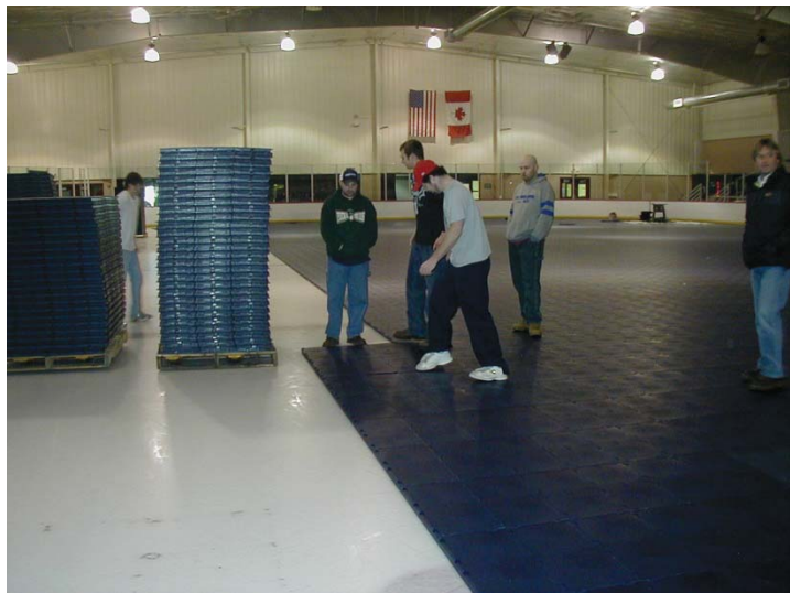
The County recently installed a dry floor at the County Civic Arena to make the facility useful for other events.
